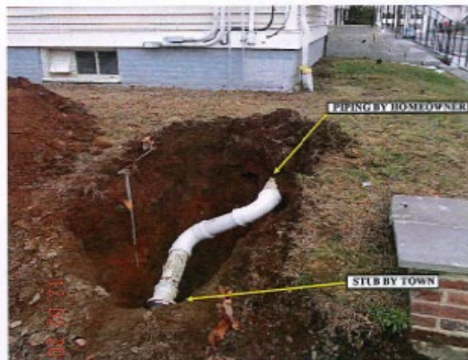
MUNICIPAL DRAIN SERVICES
